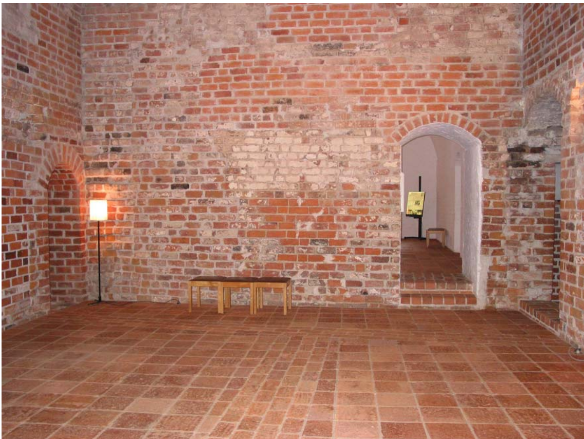
Picture 6. The eastern gable of the northeast wing. Photograph: Terhi Mikkola. (NBA, Häme Castle).
