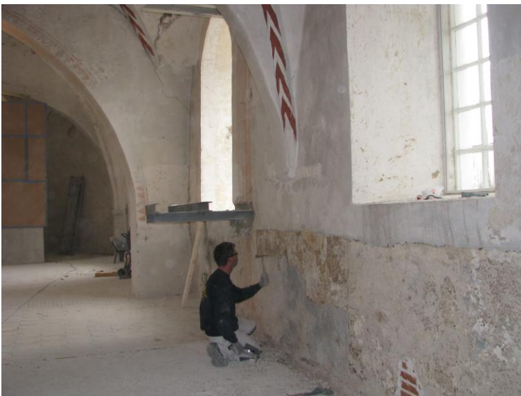
Fig. 15. Snesere church. Masons worked for weeks chipping down the wall plaster. Photo Nationalmuseet 2013.
