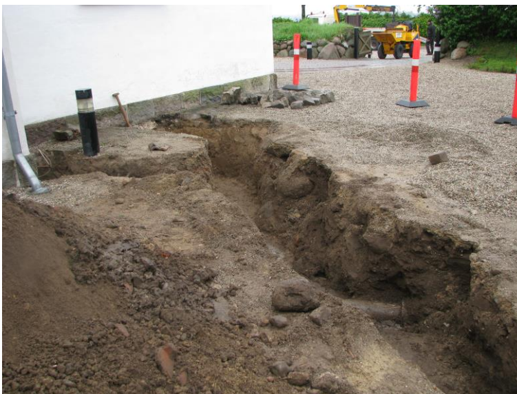
Fig. 7. Kirke Hyllinge church. Excavations on the north side of the present tower revealed two layers of stones of the foundation. The top of a third layer was seen in the bottom of the trench. Photo Nationalmuseet 2013.
