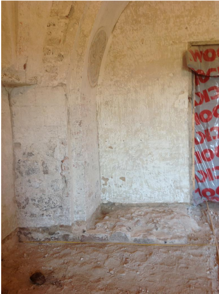
Fig. 18. Snesere church. The east wall of the Gothic tower, seen from the west. This was originally the west wall of the Romanesque tower. Only the far north (seen in the photo) and the far south ends of the fieldstone wall are preserved to one metre above present floor level, as parts of the vault pillars. The foundation of the demolished parts of the wall is preserved under the floor and could be seen during the renovation. Photo Nationalmuseet 2013.
