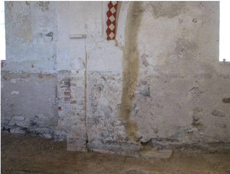
Fig. 16. Interior of the south wall of Snesere church. The original west wall of the nave (to the right) has been modified into a vault pillar in the south-east corner of the present west end of the nave. Photo Nationalmuseet 2013.
